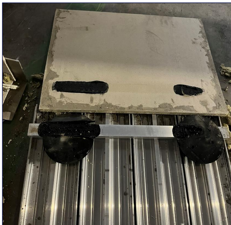
Figure 7: Damage investigation – Sample C – Pedestal and rigid foam insulation.
