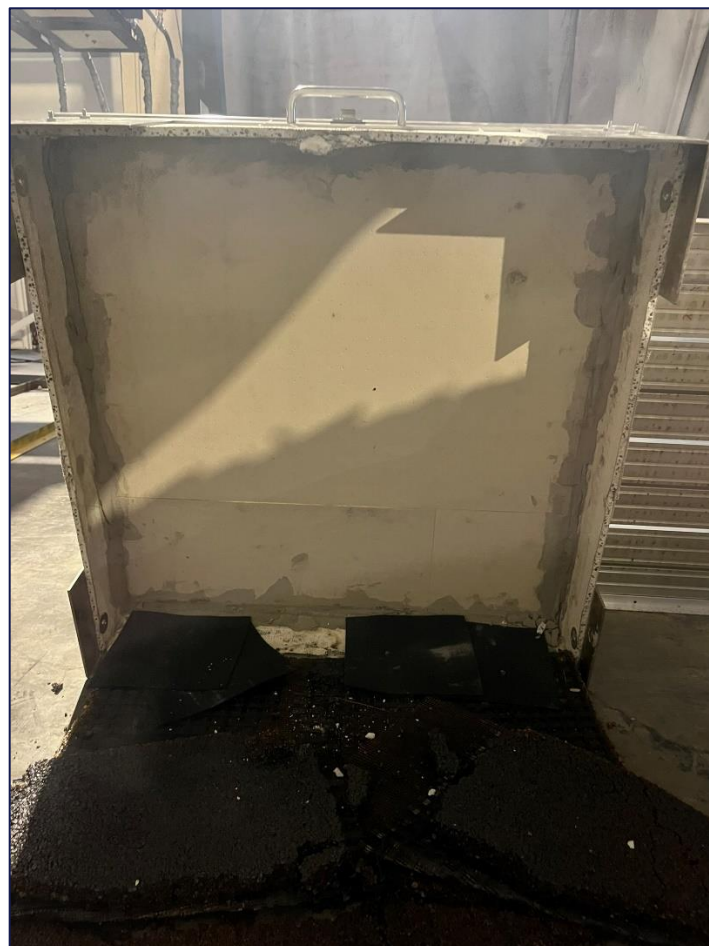
Figure 3: Air seal (mortar sealant) performed at the top of the rigid insulation foam.
