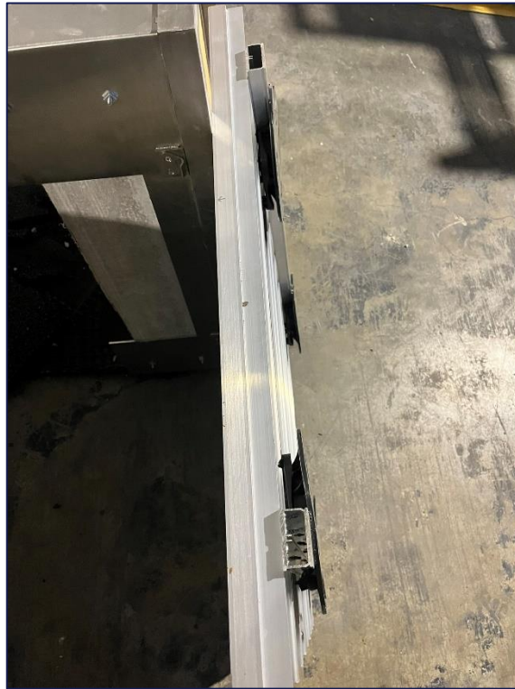
Figure 13: Damage investigation – Sample F – Pedestal.
